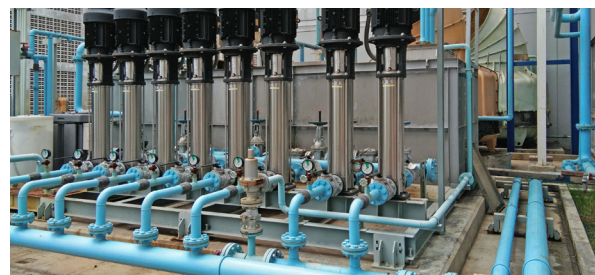
There are a variety of different inputs and controls that may be applied to the drive being used on pumping applications.
